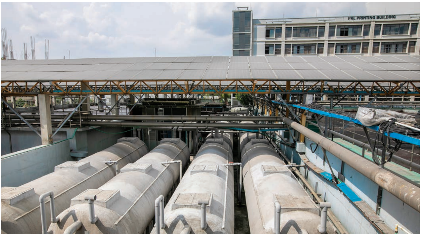
Top left: An exhaust gas absorption chiller absorbs heat and helps maintain the factory floor's temperature at around 28 °C (82 °F).
