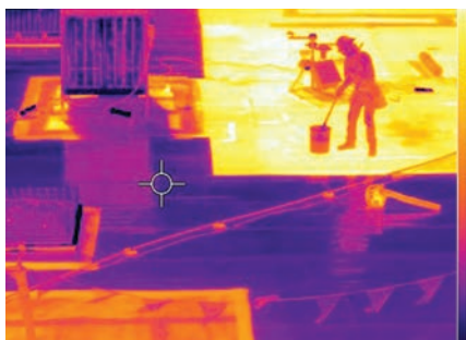
A thermal image captured during a SkyCool installation shows treated areas (white, yellow) that are roughly 35 °C cooler than the surrounding rooftop.
